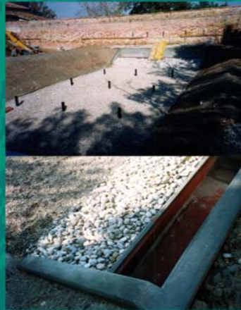
Natural wastewater treatment system
